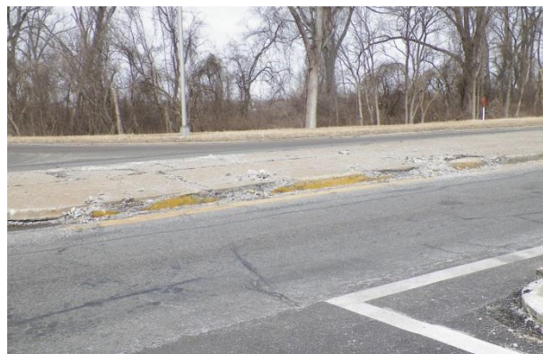
Cracked, chopped and crumbling road and median
