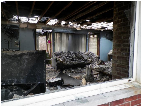
Collapsed ceiling, broken windows, exposed insulation
