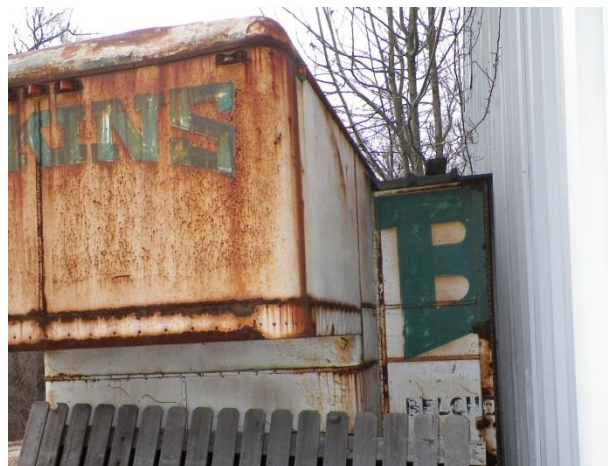
Rusted trailer attached to primary building
