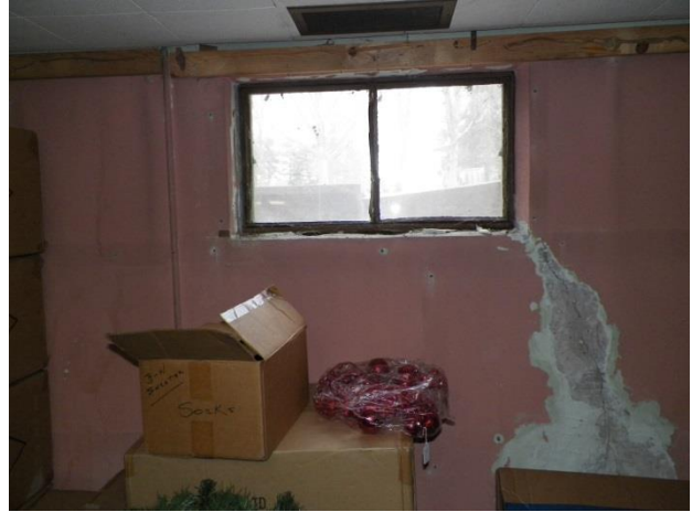
Water damage and cracks in building foundation
