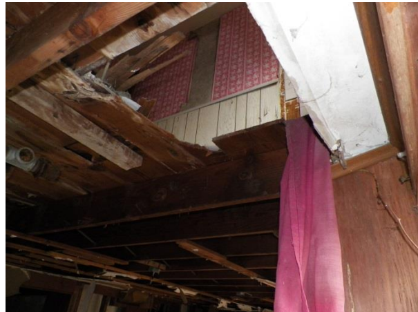
Holes in main floor of building to basement
