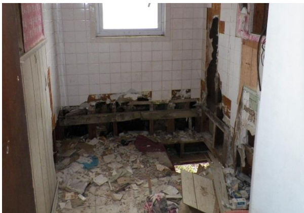
Holes in floors and exterior walls, broken tiling
