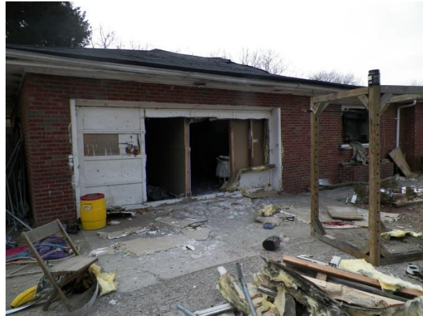
Holes in exterior walls and broken windows
