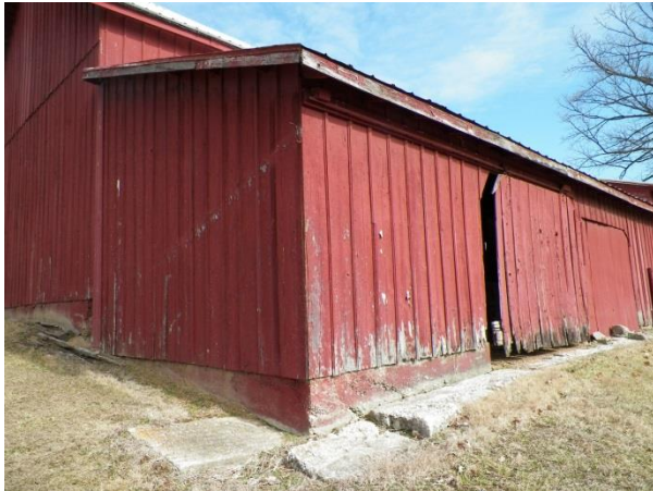
Cracked rotting wood and crumbling foundation
