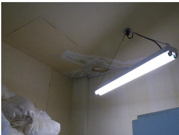
Cracked, molding and water damaged ceiling
