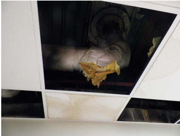
Water damage, missing ceiling tiles and torn insulation
