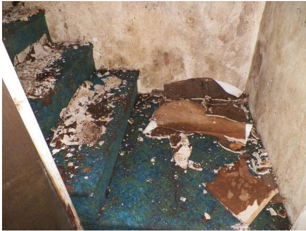
Water damage, mold/mildew and collapsed ceilings
